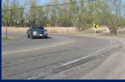
Example of fading centerline and edgeline. (Photo Source: FHWA)
